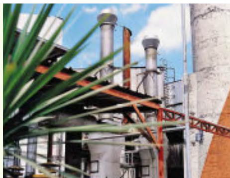
Supporting UN Global Compact Environmental Principles: Conversion from coal to gas at Nestlé's Graneros plant in Chile
